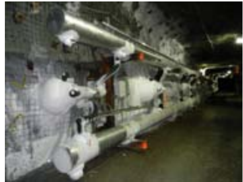
Freezing system underground at Giant Mine
