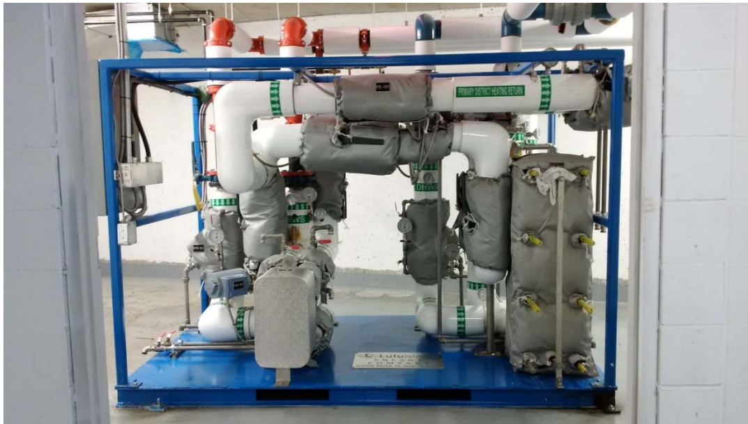
Figure 11: Typical Large Building Prefabricated Energy Transfer Station
